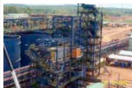
Structure for tanks
